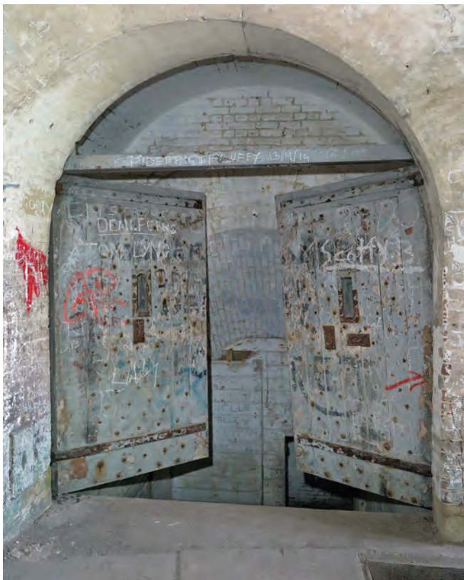
North entrance, the heavy wood and iron doors to the galleries below. Photo Clive Penfold
